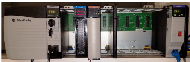
FIG. 1. ControlLogix PLC Test Station.
